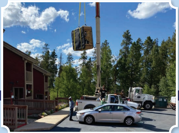
New hot tub is craned in to a condo in building C.
